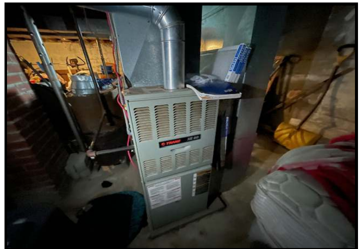
428 Government F/A Gas Furnace
