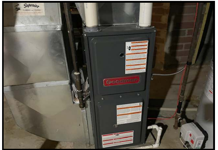
424 Government F/A Gas Furnace (2025)
